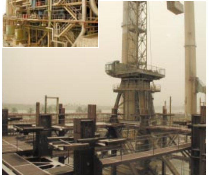
Hartha Power Station.
