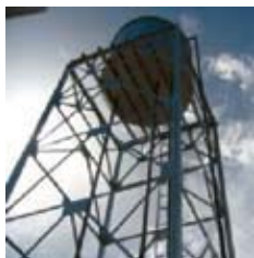
▶ Small water supply facility (elevated water tank) (Photo:JICA)
