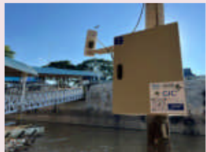
CCTV camera installed with Japan's assistance and the cooperation of the local government. Images are analyzed using artificial intelligence (AI).
