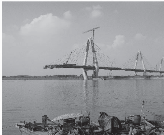
The view of the Nhat Tan Bridge during its construction from downstream of the Red River. (Photo: Yusuke Kajimura)
