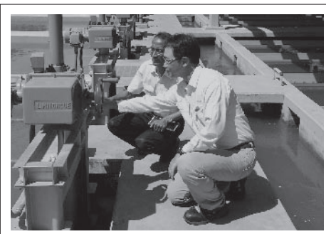
Confirmation is made about the valve update plan with the manager in charge of water purification at the Phum Prek Water Treatment Plant in Phnom Penh. (Photo: Takayuki Kawasaki)
