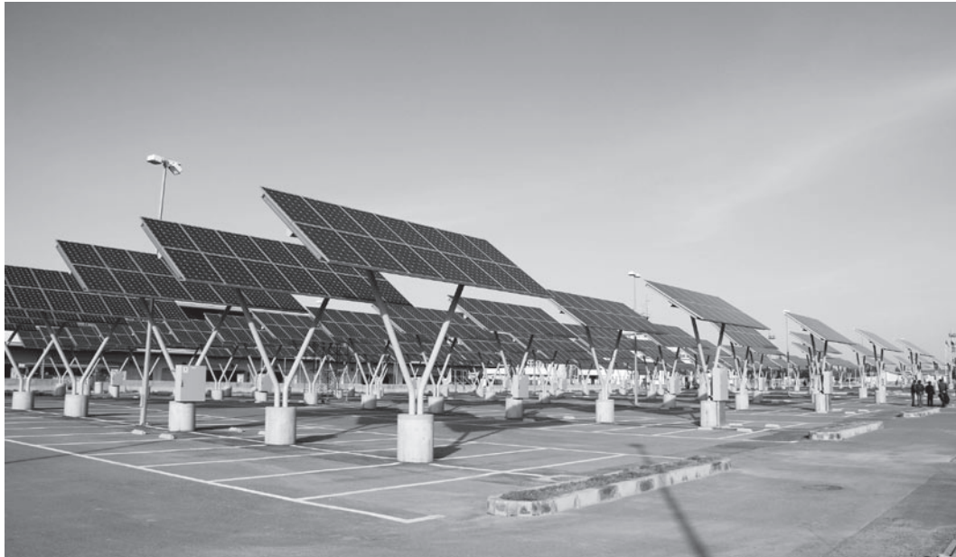
A grid-connected photovoltaic power generation system was installed at the Kabul International Airport facility in Afghanistan. Approximately 35% of electricity demand of the international terminals is provided by this system. (Photo: Sayad Jan Sabawoon / JICA)
