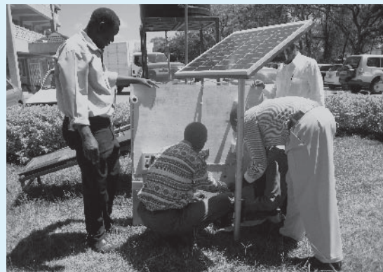
Project for Capacity Development for Promoting Rural Electrification Using Renewable Energy (Photo: JICA)
