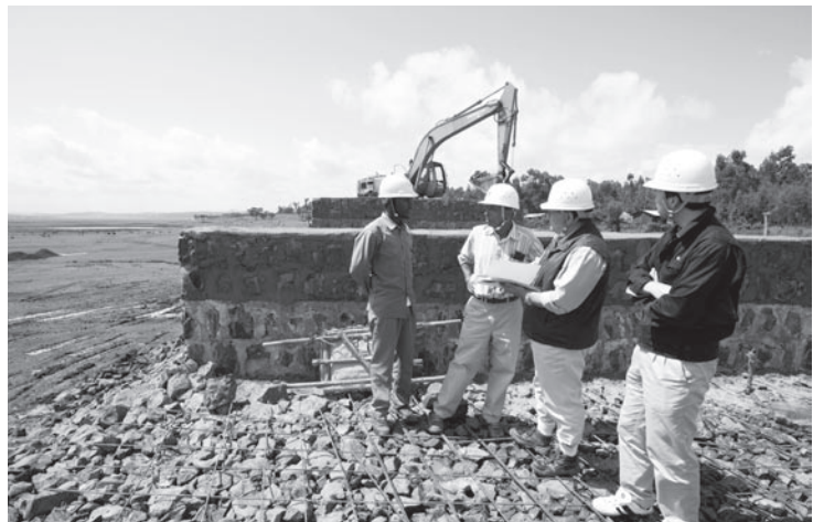
Japanese engineers who are building a construction camp as part of the Project for Rehabilitation of Trunk Road, Phase 4 in Ethiopia (Photo: Kenshiro Imamura / JICA)
