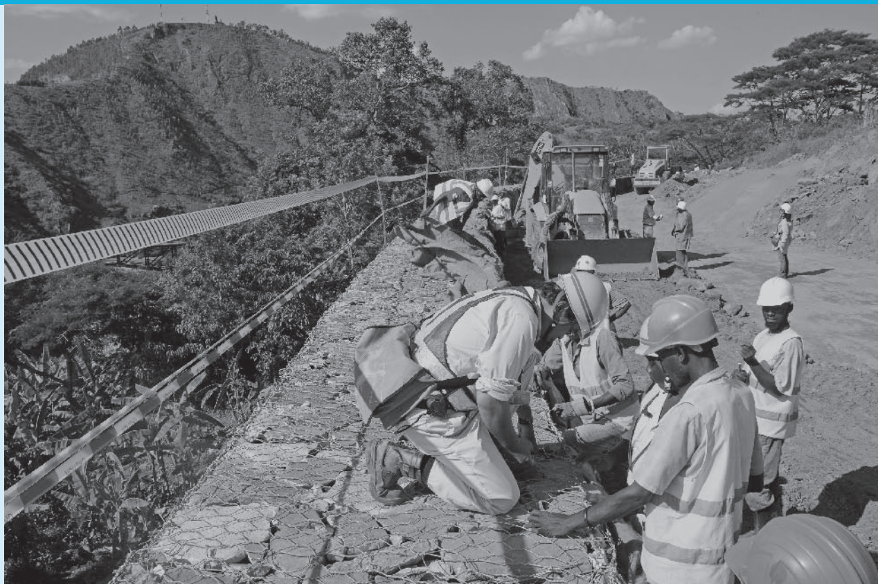
A Japanese engineer working and giving guidance at the Rusumo International Bridge that connects Tanzania and Rwanda (Photo: Takeshi Kuno / JICA)
