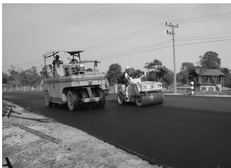
A project to improve roadway maintenance capabilities in Laos. Repairs were done in badly damaged areas. (Photo: JICA/International Development Center of Japan/Oriental Consultants)
