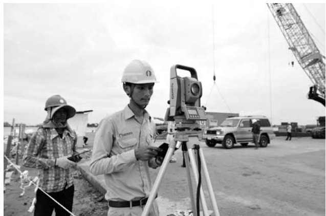
Project for Construction of Neak Loeung Bridge in Cambodia Vietnamese engineers survey the planned site for construction of the Neak Loeung Bridge. (Photo: Koji Sato/JICA)
