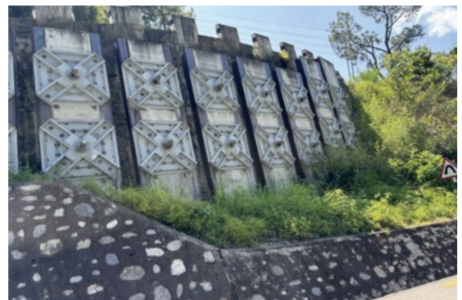
Slope stabilization done by the Project for the Rehabilitation of Sindhuli Road after the 2015 earthquake (Photo: Evaluation Team)
