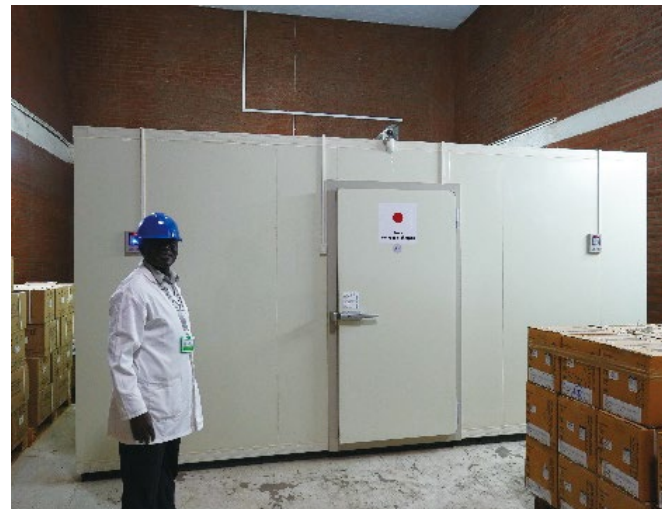
Cold room provided to the central pharmaceutical warehouse in Malawi (Photo: Evaluation Team)
