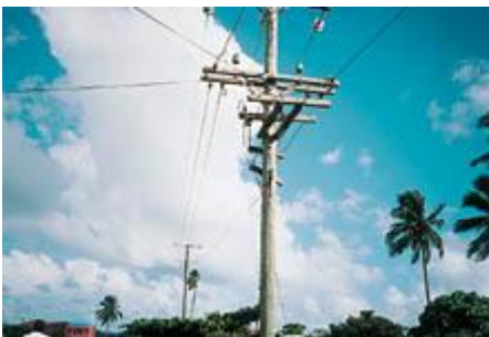
Power cables (upper ones) and telephone cables (lower ones)
