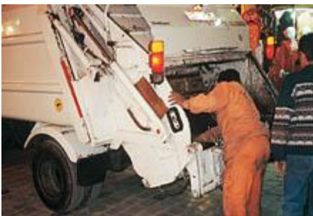
Refuse Disposal Equipment Improvement Project in Damascus: refuse collection work in progress
