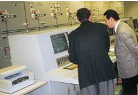
Jandar Thermal Power Station Construction Project: control room
