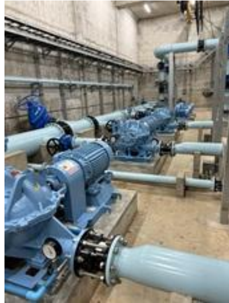
Right photo: Water treatment plant (pump group) (Source: Photographed by the evaluation team during the Field Survey)
