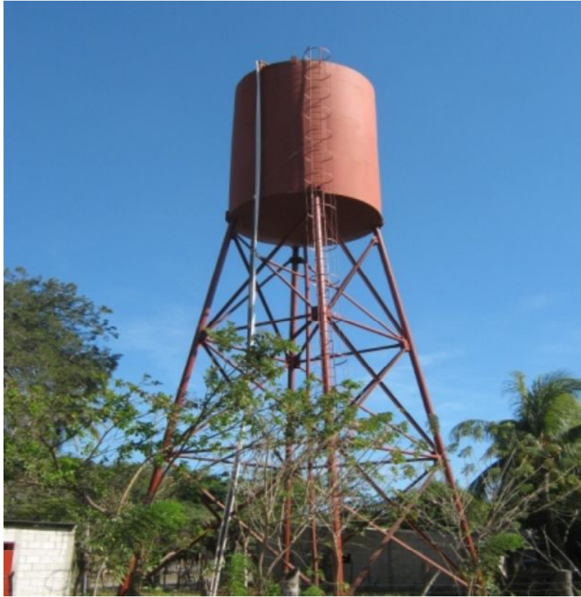
Elevated cistern (Grant Assistance for Grassroots Human Security Projects)
