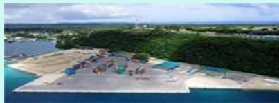
Development of the port of Port Vila in Vanuatu (Photo provided by: TOA CORPORATION)
