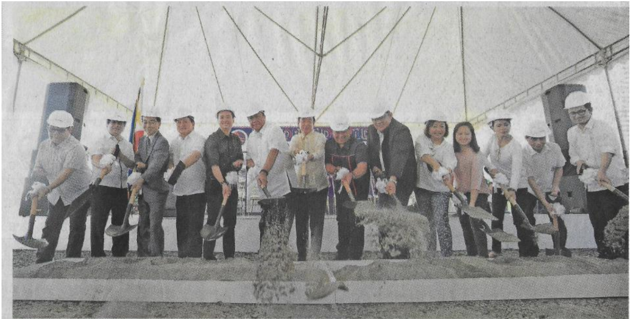
MANILA-CLARK RAILWAY PROJECT BEGINS One of the biggest infrastructure projects of the Duterte administration, the Manila-Clark Railway Project, has officially begun, as the Department of Transportation leads the groundbreaking rites of the first phase of the ambitious project that links Metro Manila to Clark in Pampanga. The groundbreaking ceremony was held at an open area in Maria Socorro, Marilao, Bulacan, and was led by Transportation Secretary Arthur Tugade, Senators Joel Villanueva and JV Ejercito and other national and local officials. The landmark project will help ease vehicular traffic in Metro Manila and speed up travel from Manila to Clark to only an hour. Rail stations will be strategically located in key growth areas from Manila, Bulacan and all the way to Pampanga. Photo shows (from left) Philippine National Railways (PNR) Chairman Gen. Roberto Lastimoso, Meycauayan Mayor Henry Villarica, Japan International Cooperation Agency Chief Representative Susumo Ito, Bulacan Gov. Wilhelmino Sy-Alvarado, Villanueva, Tugade, Japanese Ambassador Koji Haneda, Ejercito, PNR General Manager Jun Magno, Bulacan 4th District Rep. Linabelle Villarica, Bocaue Mayor Eleanor J. Villaenueva-Tugna, Marilao Mayor Juanito Santiago and Bases Conversion and Development Authority President Vince Dizon.
