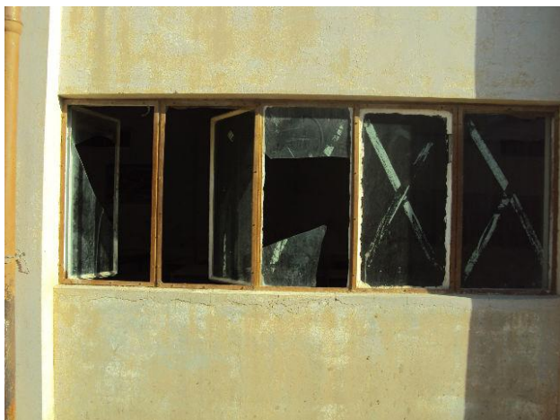
教室の窓修復前 (Al-Hayat school)
