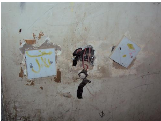
校内電気設備修復前 (Al-Hayat school)
