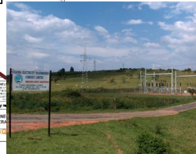
Mbarara North Substation
