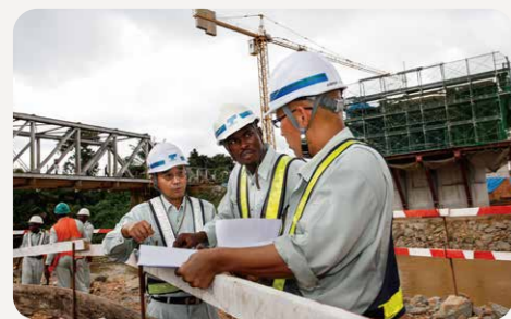
Rehabilitation made on National Trunk Road No.8 in Ghana Photo credit: Akio Iizuka
