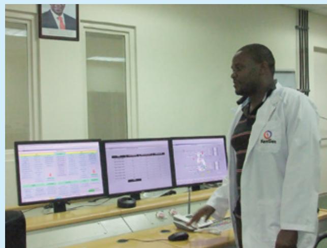
Control room of the geothermal power plant in Olkaria (Photo by JICA)
