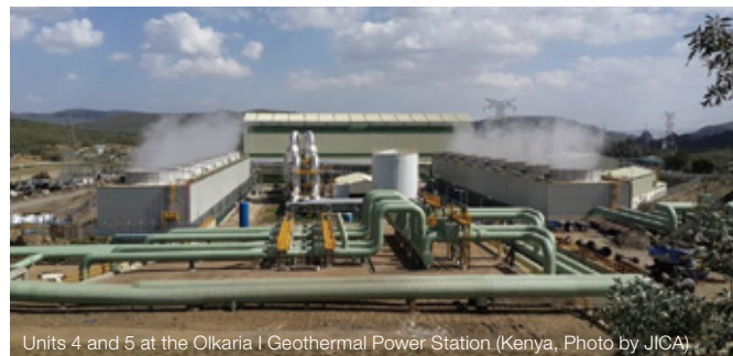
Units 4 and 5 at the Olkaria I Geothermal Power Station (Kenya, Photo by JICA)
