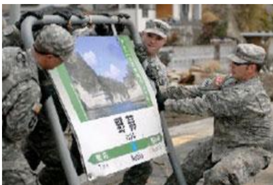
The U.S. Army engaging in repair operations on the railroad at Nobiru Station on the Senseki Line (Higashi Matsushima City) (U.S. Army Photo)
