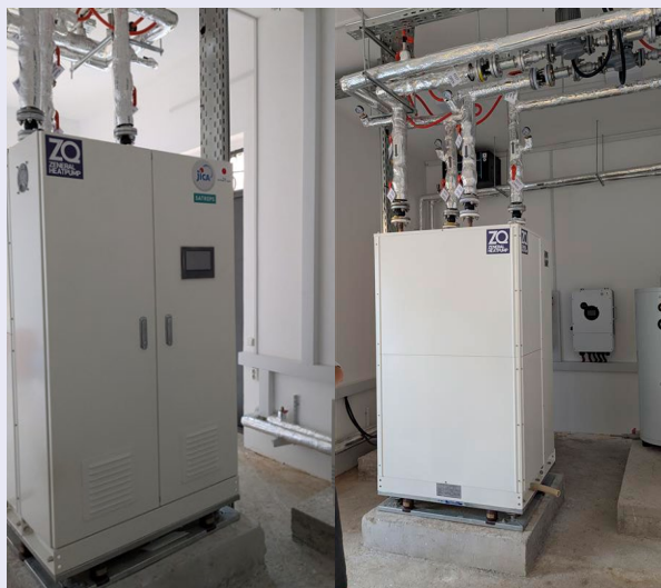
GSHP system installed at the first demonstration site (Dushanbe) (Photo: Akita University)
