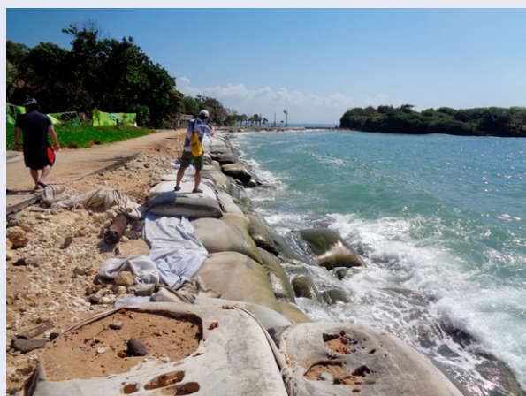
Nusa Dua Beach before the project, with visible damage and collapse of the seawall (Photo: Nippon Koei Co., Ltd.)
