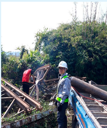
Dr. Thavone confirming the strength of the components of a collapsed Bailey bridge, as part of his research activities in Laos (Photo: Nagasaki University)
