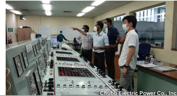
Chubu Electric Power Co., Inc
