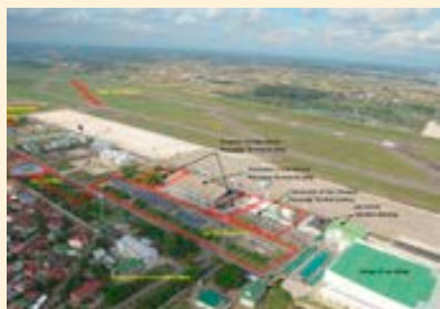
Construction area of this project (Construction area is shown with the red line, 2014) (Photo: Hazama Ando Corporation)
