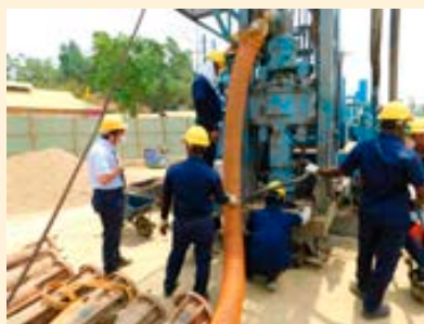
Deep-well drilling operation at the camp for displaced persons from Myanmar in Bangladesh (Photo: JICA)
