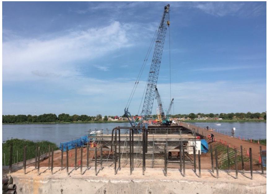
Bridge construction work in progress across the Nile in Juba (courtesy of JICA)
