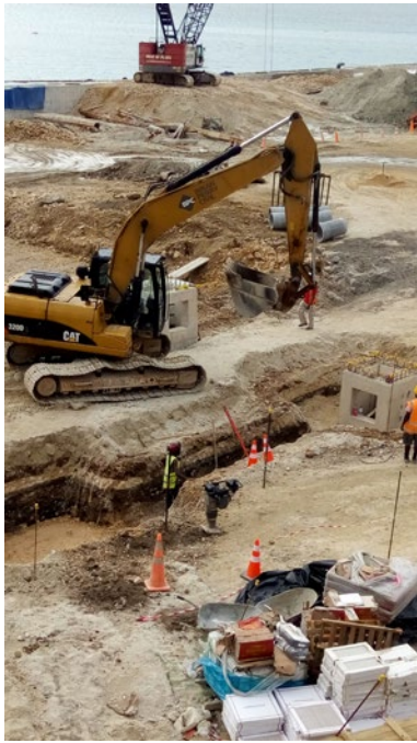
Site of the Port Vila Lapetasi International Wharf Development Project in Vanuatu. Excavation works are carried out for the installation of drainage pipes. (Photo: Mr. Takeda / ECOH CORPORATION)
