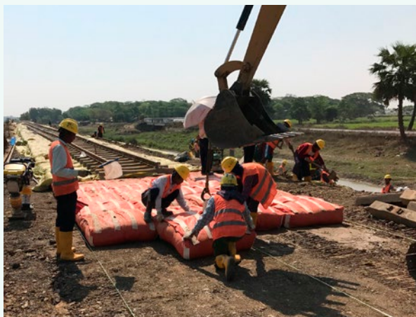
Laying D-Box sandbags for the construction of a railway line in Myanmar (Photo: Mety Co., Ltd.)
