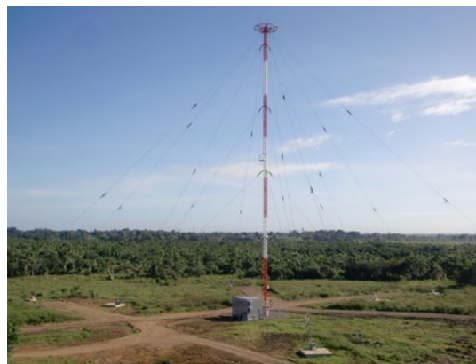
An antenna for medium wave radio broadcasting (Photo: JICA)
