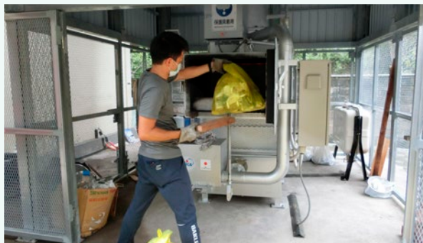
Garbage being inserted into the Chirimeser, small-sized incinerator (Photo: Thomas Technical Institute Co., Ltd.)
