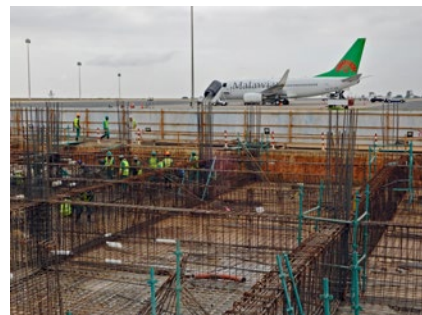
The foundation frame construction site of the international passenger terminal arrival wing (Photo: GYROS Corporation)
