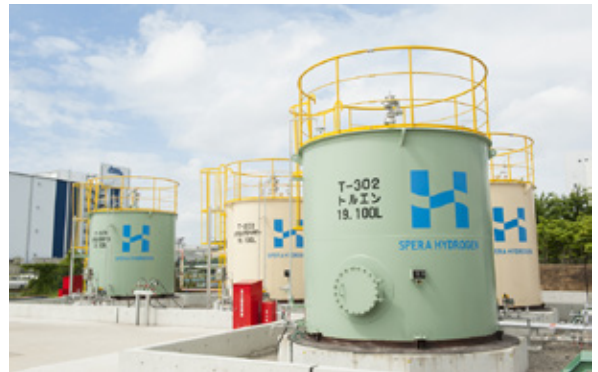
Storage section in the SPERA Hydrogen® demonstration plant at Chiyoda’s R&D Center in Yokohama Courtesy of Chiyoda Corporation
