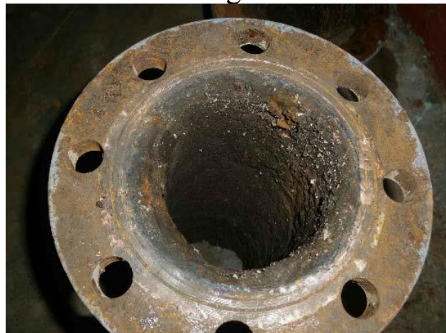
Substance accumulated on pipes
