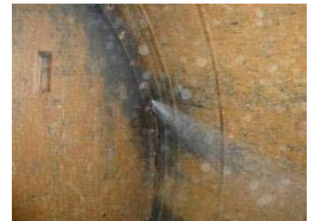
Leak from the input valve of the water wheel
