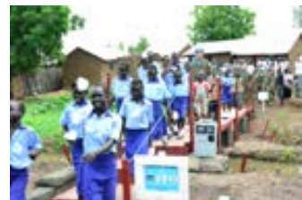
Crossover bridge constructed by the Self-Defense Force at an elementary school in the Republic of South Sudan
