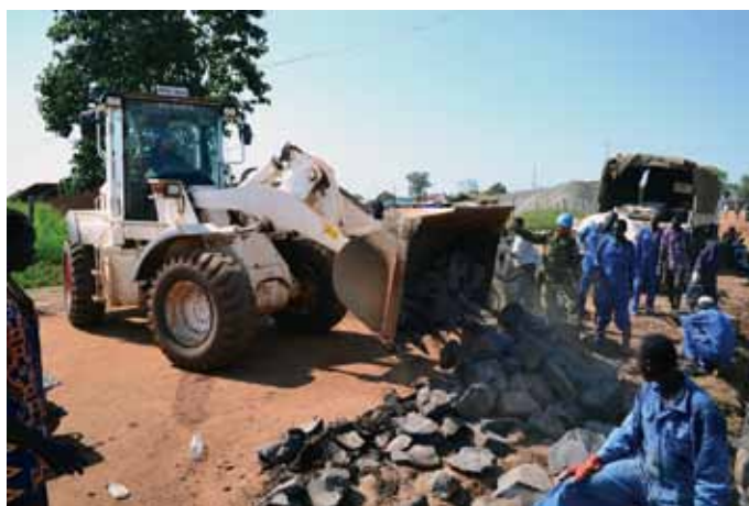
A Self-Defense Forces Engineer Company working together with local citizens to build a community road in the Na-Bari district of the capital, Juba, in coordination with Japan's ODA project under the UN Mission in South Sudan (UNMISS) (South Sudan; Source: Ministry of Defense)
