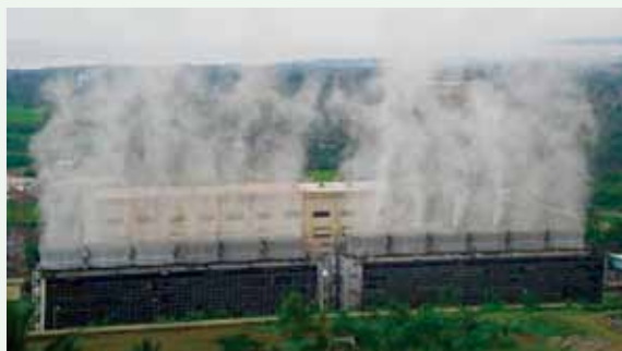
Tiwi Geothermal Power Plant
