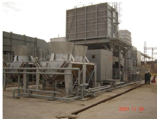
Constructed power-generating plant
