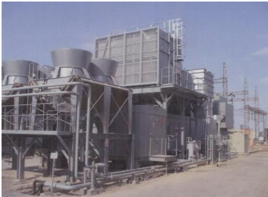
Completed power-generating plant No.5
