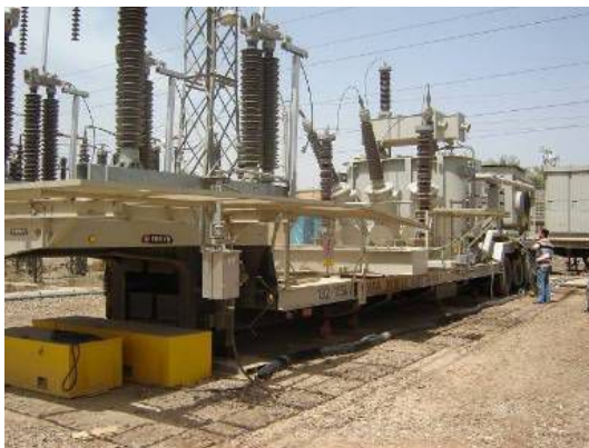
Substation facilities set up in Iskan Al Kher
