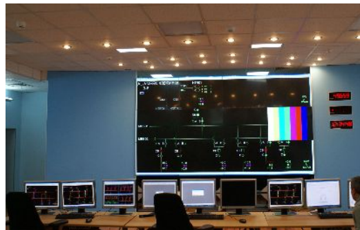
Control room after renovation
