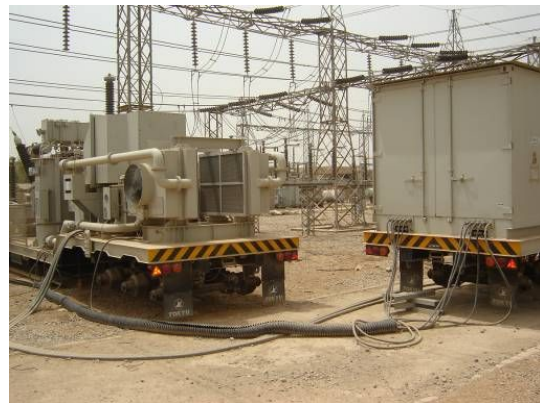
Substation facilities set up in Rashidiya
